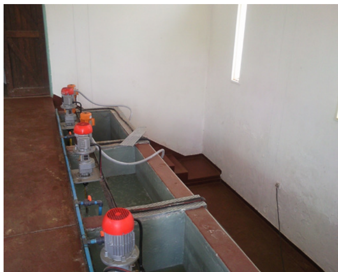
Bindura. Chemical dosing system after rehabilitation
