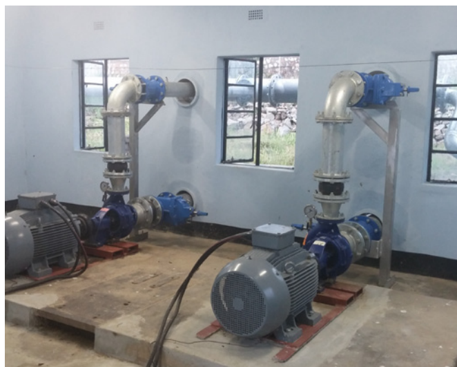
Plumtree. Mhlanga high lift pump station after rehabilitation
