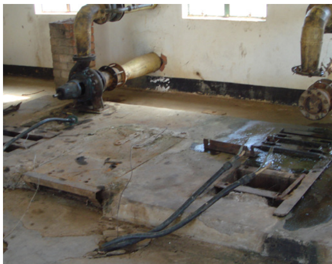
Plumtree. Mhlanga high lift pump station before rehabilitation
