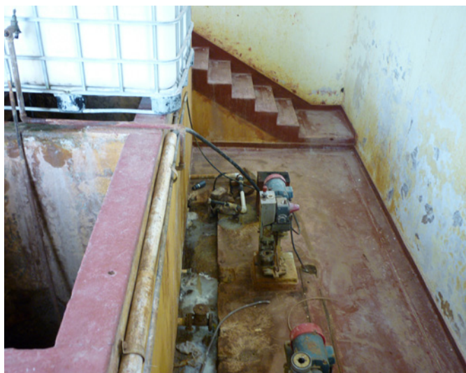
Bindura. Chemical dosing system before rehabilitation
